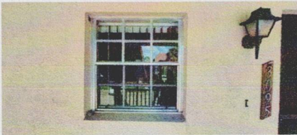
Unprotected glazed opening
