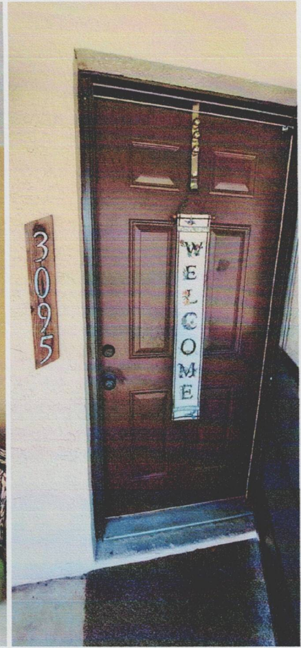
Unprotected non-glazed entry door
